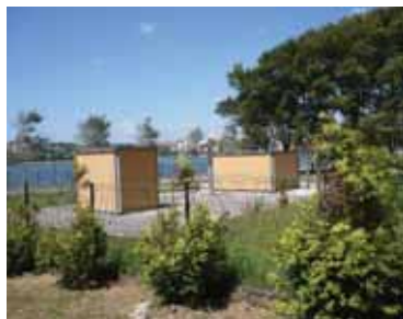
Afurada pumping station. The system showed significant pump efficiency deterioration, so the impellers were replaced.
